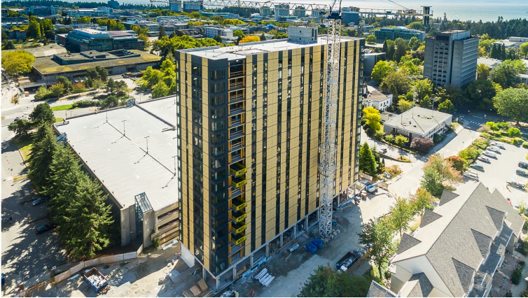
Figure 23. An 18-story hybrid mass timber residence at the University of British Columbia (UBC). Source: http://news.ubc.ca .
