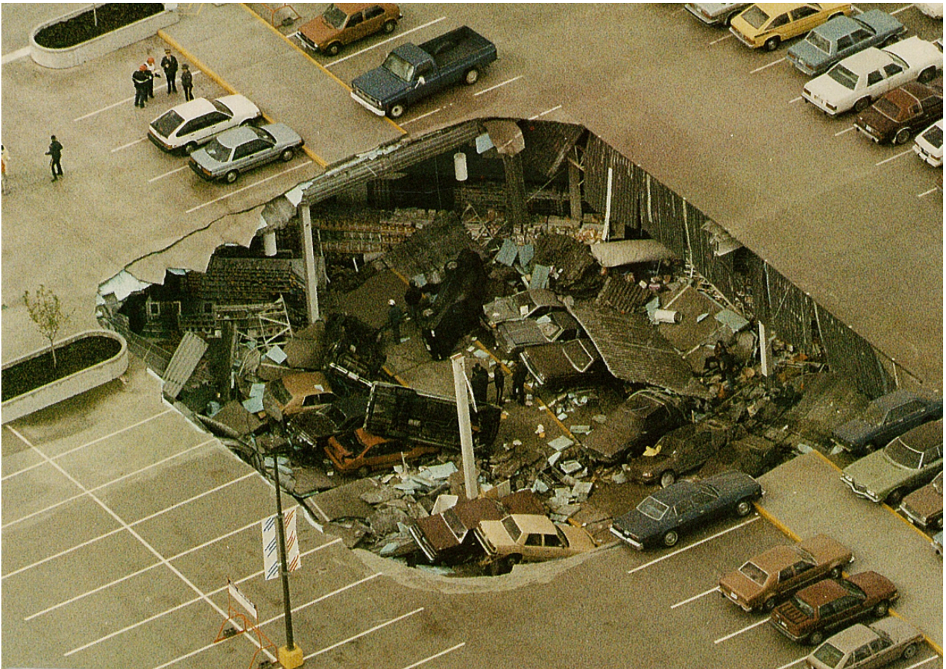
The roof top parkade of Save-on-Foods collapsed in Burnaby in 1988
