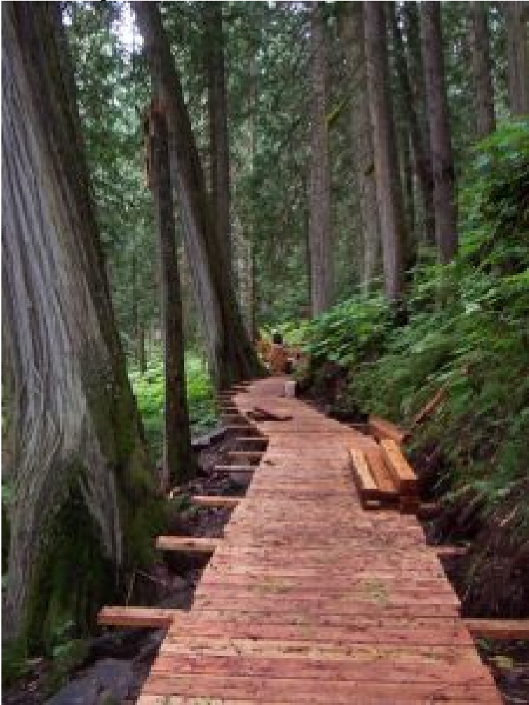
Figure 8. Nowell Senior Universal Boardwalk under construction, part of the Ancient Forest Trail.
