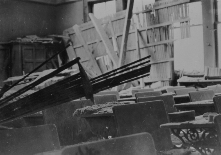
Figure 11.1 A schoolroom in Courtenay damaged by the 1946 Vancouver Island earthquake. If the earthquake had not happened on a Sunday, the casualties would have been much greater. [from Earthquakes Canada, http://www.earthquakes.canada.nrcan.gc.ca/historic-historique/events/images/19460623_1946.school.inside.jpg ]
