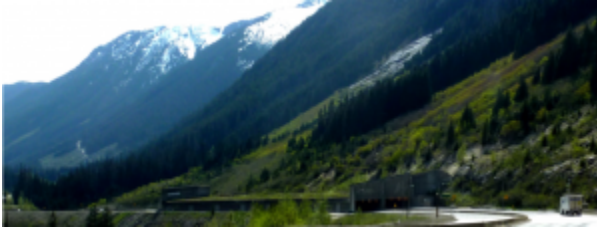
Figure 15.21 A snow avalanche shelter on the Coquihalla Highway. The expected path of the avalanche is the steep un-treed slope above. [SE]
