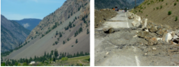
Figure 15.8 Left: A talus slope near Keremeos, B.C., formed by rock fall from the cliffs above. Right: The results of a rock fall onto a highway west of Keremeos in December 2014. [SE]
